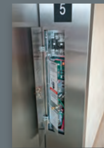
D INSPECTION & TEST PANEL Most necessary test and maintenance features are concealed behind a panel in the elevator entrance.
